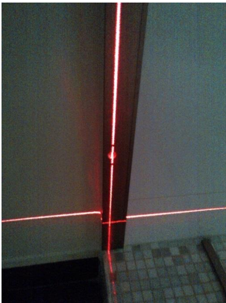
Perfect alignment of the glued profile along the vertical traced by the laser.
